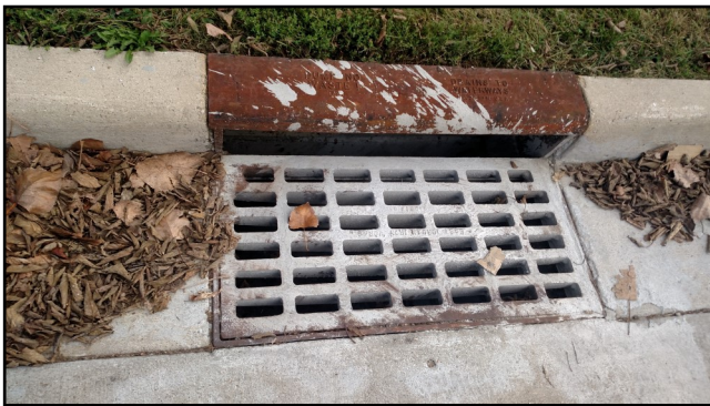
Build-up of leaves and staining from an illicit discharge on storm drain.
