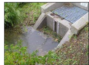
Trash grate on side and top
