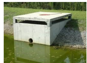
Outlet with low flow orifice
